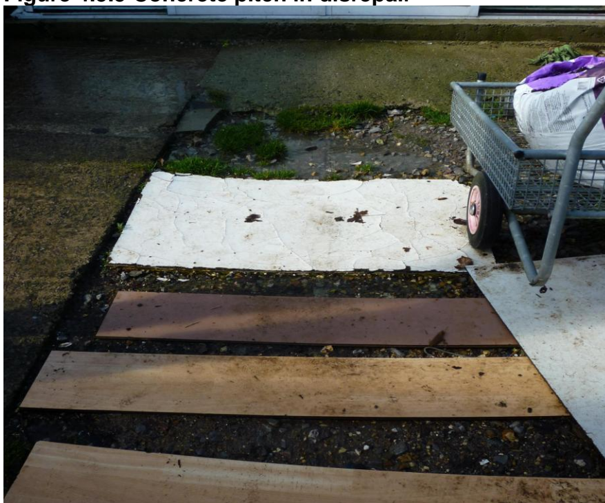
Figure 4.5.5 Concrete pitch in disrepair
