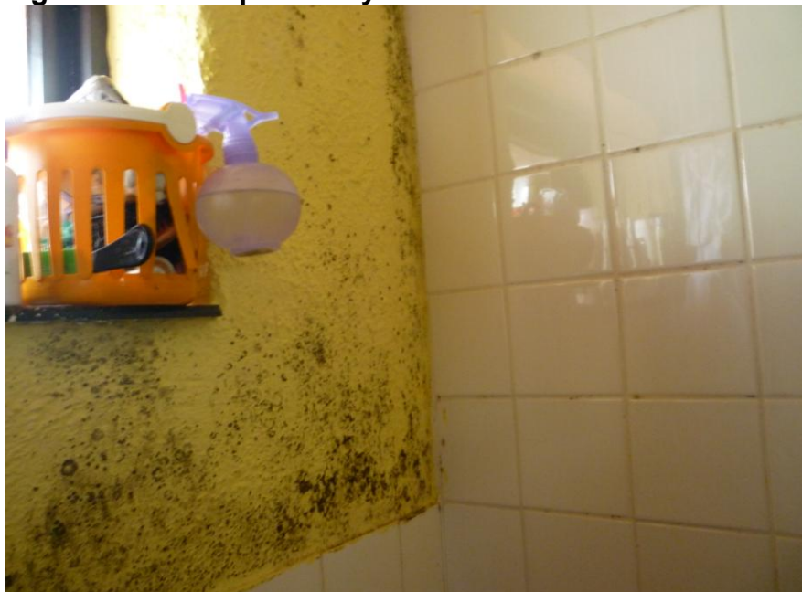
Figure 4.5.4 Damp in utility block
